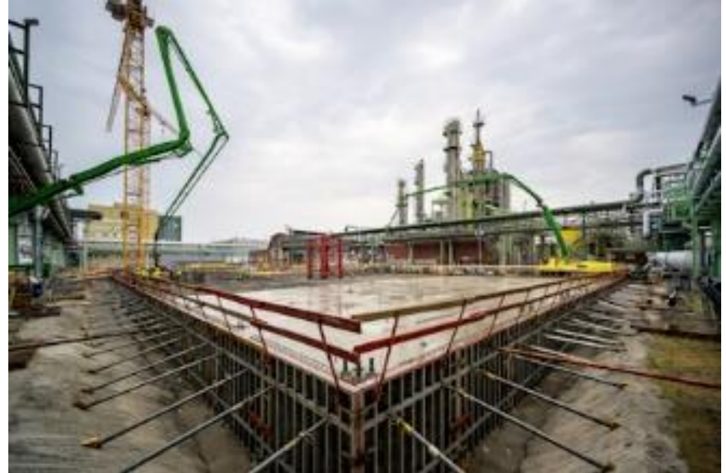
Boiler house base plate
